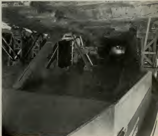
Engineers redesigned the type of blocking to be used and constructed a series of timber-braced cribs about 6 ft. 4 inches wide and 16 inches thick. These are secured to the tops of the bilge blocks and are tied together as a unit fore and aft and braced diagonally.
